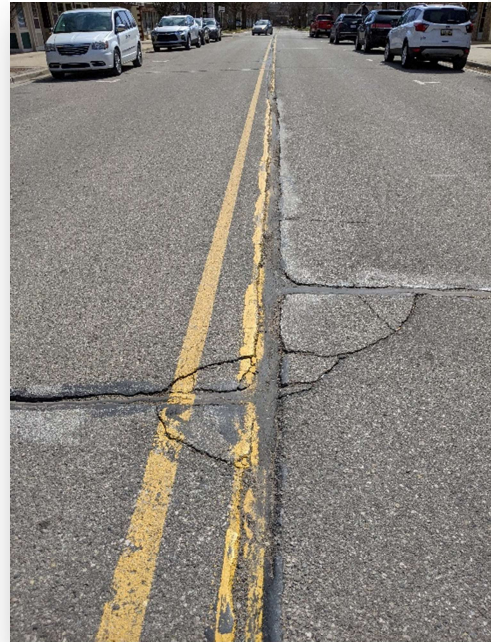
Photo 1 - Longitudinal Centerline Crack
